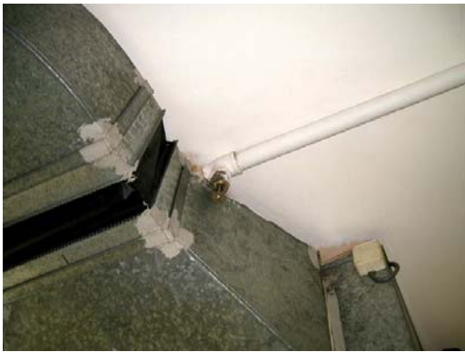
Duct degrades sprinkler coverage
