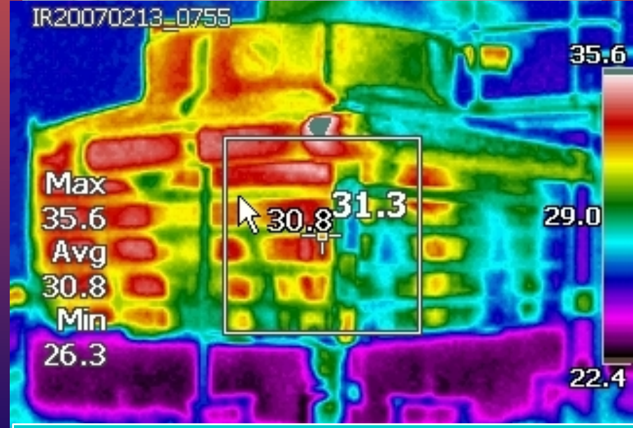
Cooling tower RMP assessment
